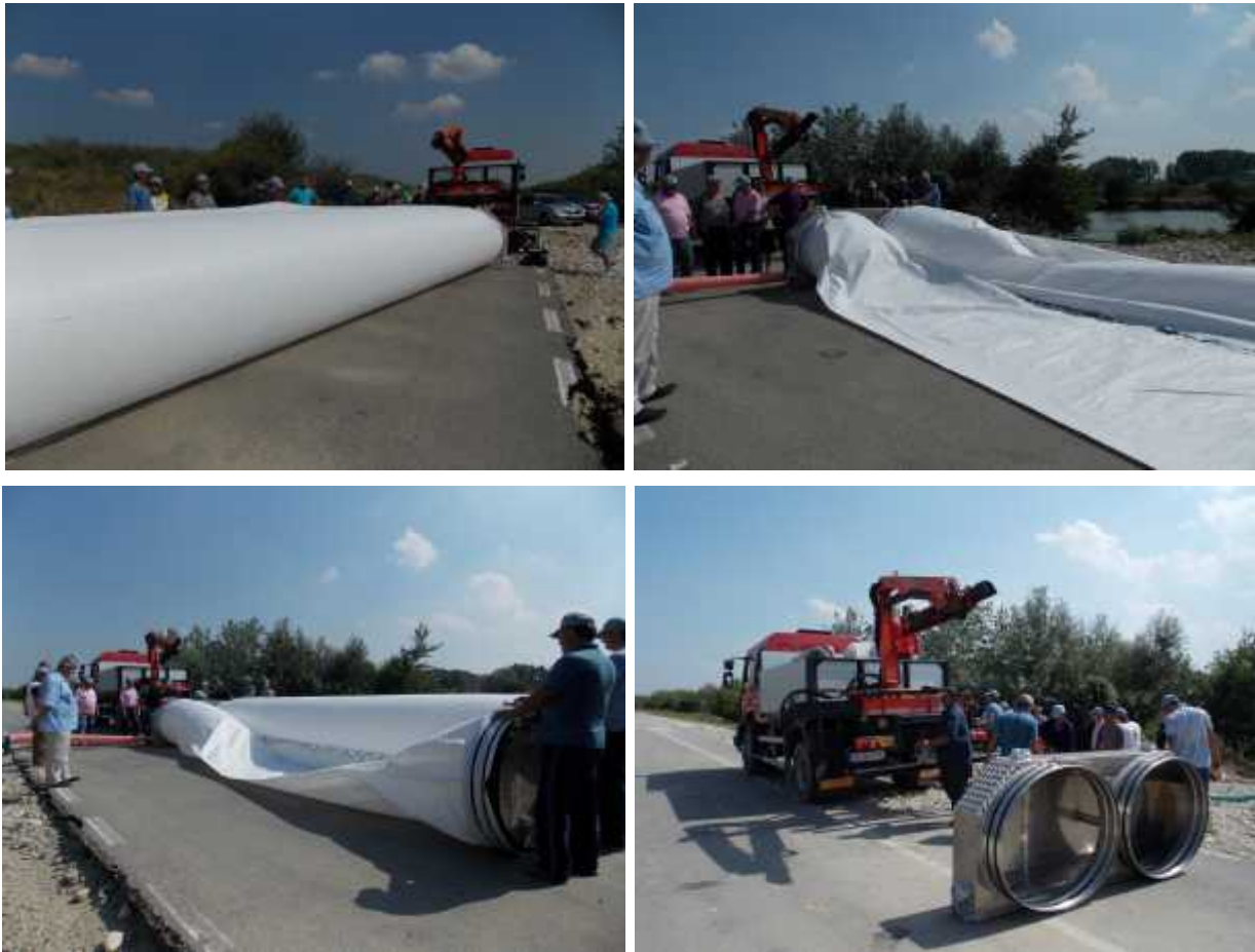
Figure 9. Mobile flood barriers
